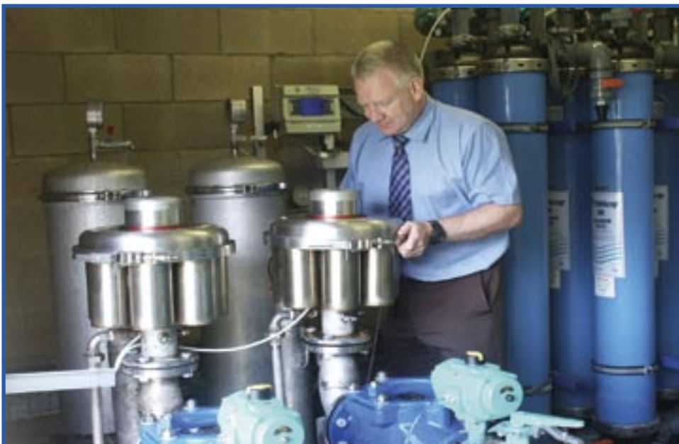
Northumbrian Water acceptance manager Tony Bell notes backwash counts on the two Cross Phoenix filters installed at Birch Tree.
