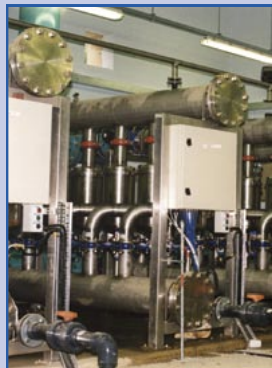
Cross 'zero gravity' filtration secures improved water
