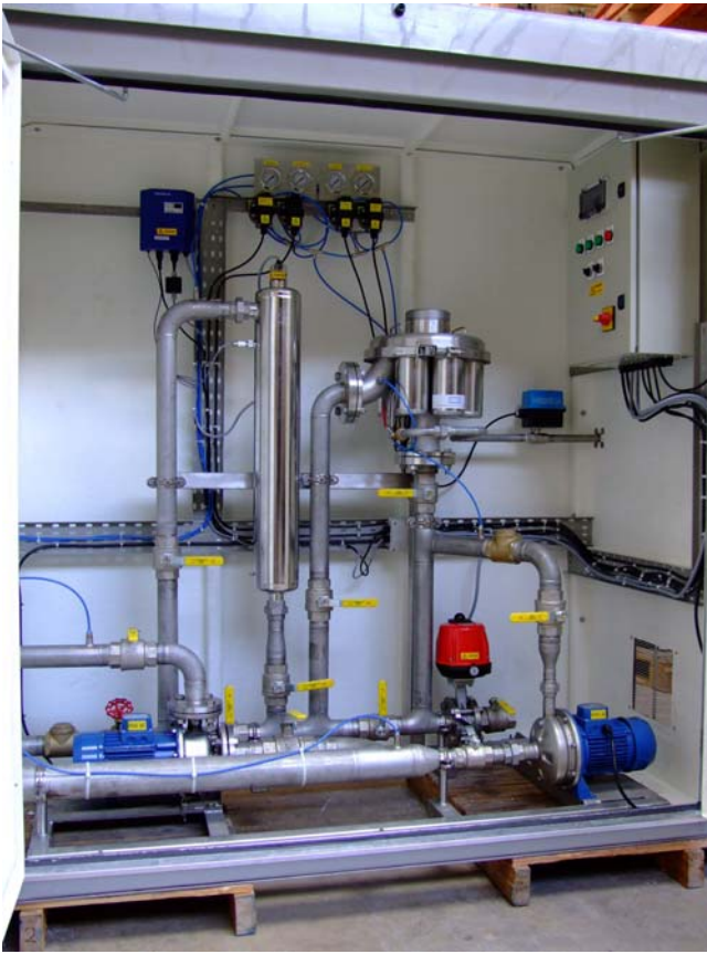
Main components of the package, left to right: Vehicle filling pump Ultra-Violet disinfection tube Cross Phoenix automatic filter Inlet isolating valve (red actuator) Re-circulating circuit pump Control panel
