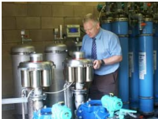
Northumbrian Water acceptance manager Tony Bell notes backwash counts on the two Cross Phoenix filters installed at Birch Tree.
